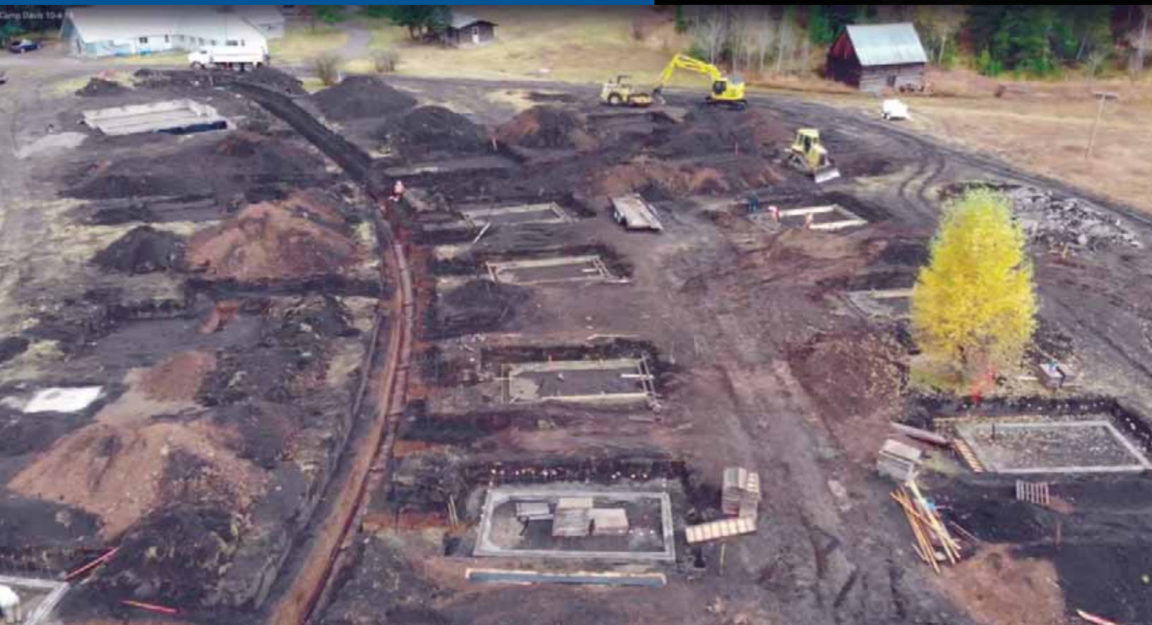
Above: New foundations are being poured for the student cabins (center and right rows), while the foundation for the new student recreation building, to replace Johnston Hall, can be seen at the upper left of the photo, near the dining hall.
